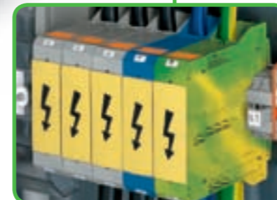
Protective warning marker may indicate: Attention! Voltage may be present despite main circuit being switched off!
